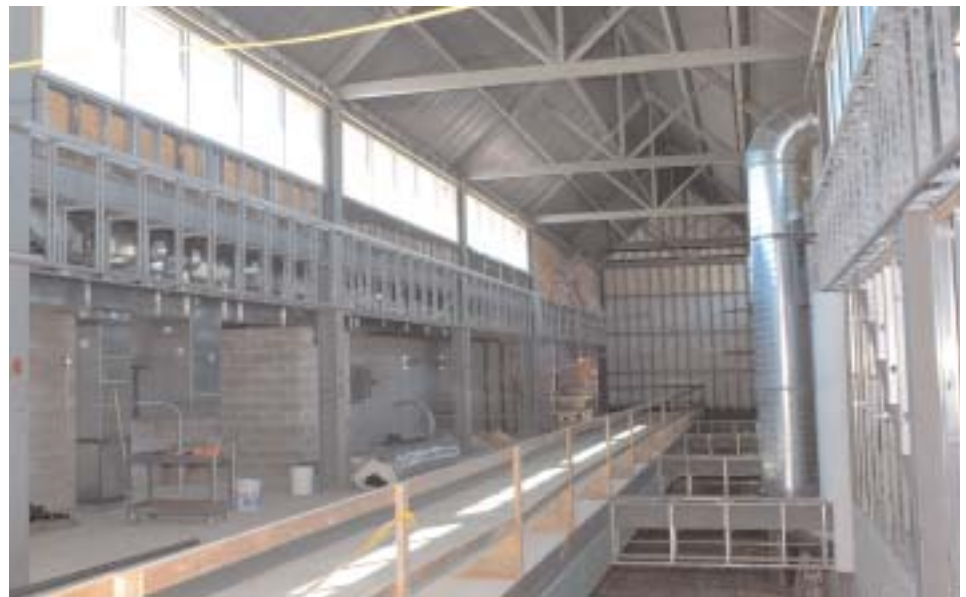
The second floor promenade will feature lots of natural light, comfortable seating areas, a decorative railing, and exposure to the first floor corridor.
